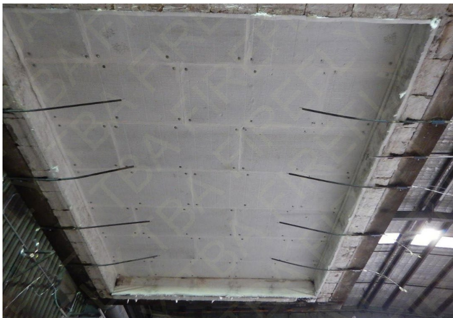
Figure 4 - Test specimen with 1200 x 600 x 500mm TBA Firefly™ Intubatt® installed – ready for 240 minutes exposure (Warringtonfire FRT210062)
