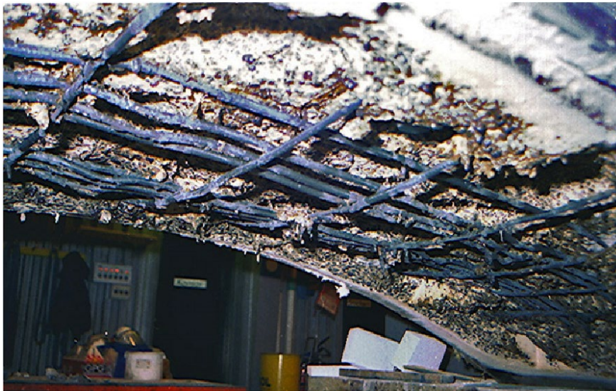
Figure 1 - Unprotected concrete structural failure: exposure of steel reinforcing due to concrete spalling – (Fire spalling of concrete – A historical overview, Robert E. Jansson 2013).
